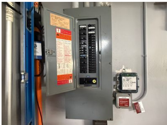
Photo Inside Electrical Panel
